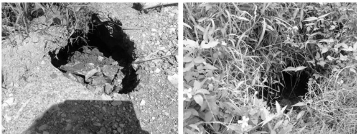
Fig. 11. Sinkholes at K21+900 positions on the Dao River right dam in Nam Định.
