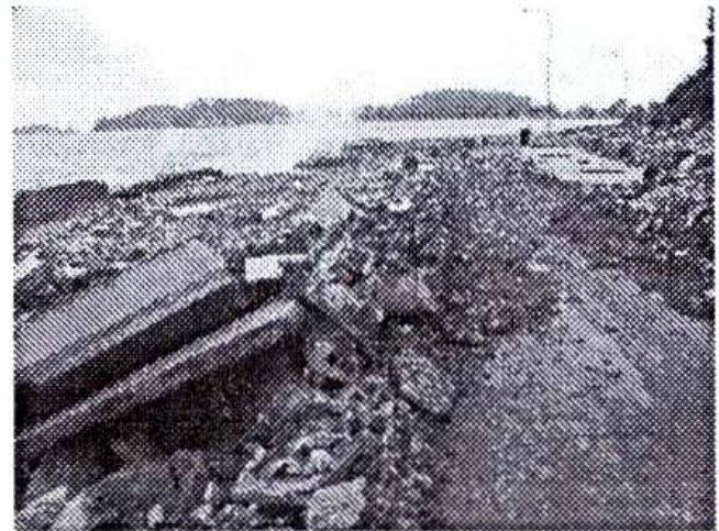
Photo 6. The destroyed infrastructure by Storm No. 7, September 2005.
