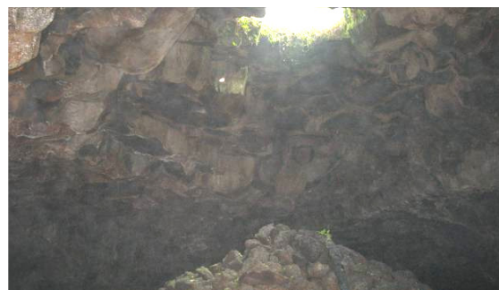
Fig. 6 Ceiling collapse of shallow cave in Choah Village (Source: La The Phuc, 2012).
