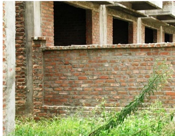
Figure 2. Cracks on Van Quan houses.
