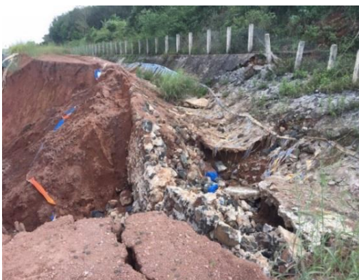
Figure 3. 2019 landslide on a road along the red mud basin No. 2 - Nhan Co alumina factory.
